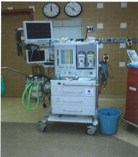
On-Site Visit: Front view of Anesthesia Machine No.1
